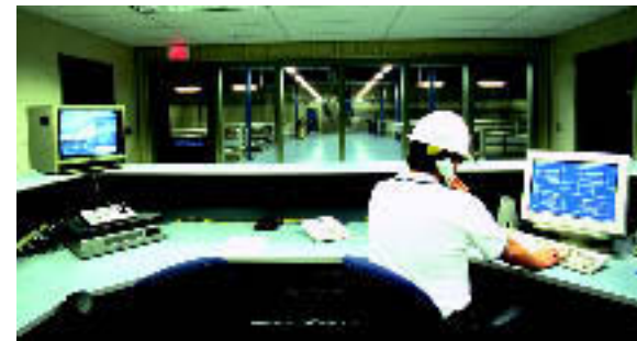
Control room at the Water Treatment Plant
